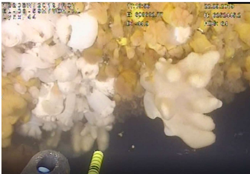
Figure 6-15 Example of marine growth on jacket.
